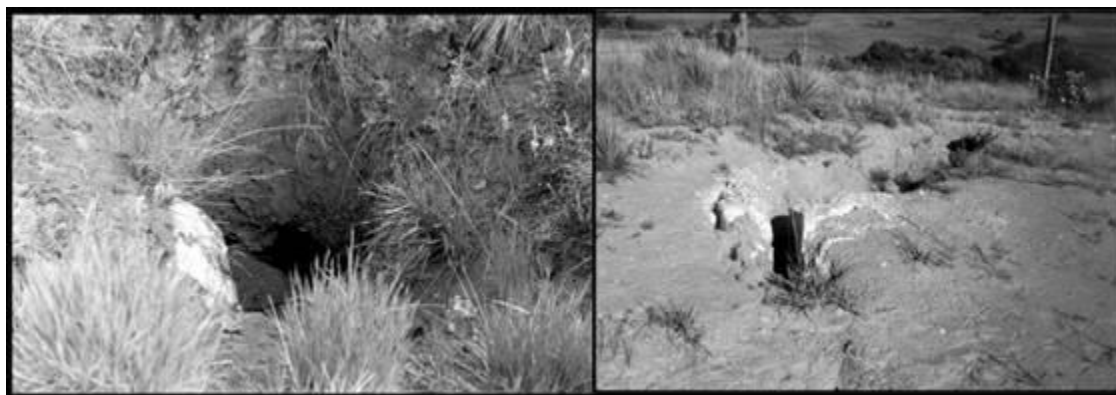
Figure 18. Many small sinkholes are present in the McNenny Fish Hatchery area, including circular depressions in red beds with some remaining gypsum (left) and solution widening of joint in gypsum resulting in soil collapse in residential parking area (right).
